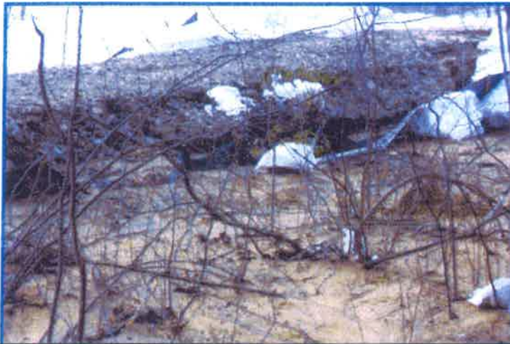
Sediment deposition within wetland on south side of roadway
