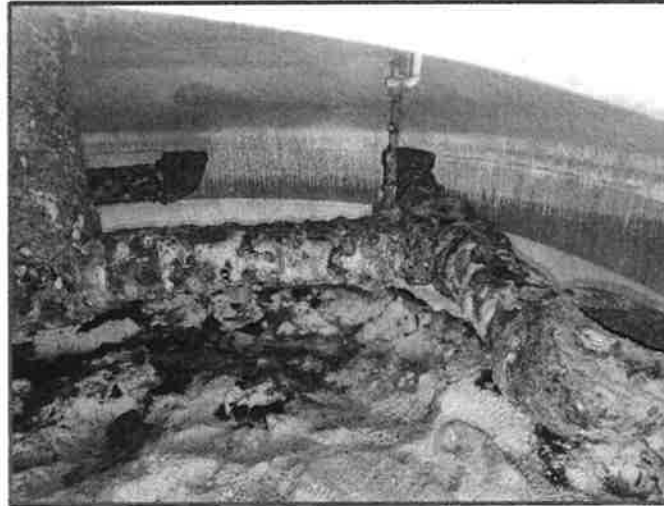
Figure 2: Inlet distributor with tuberculation and calcium-based filter media in GAC Contactor #1
