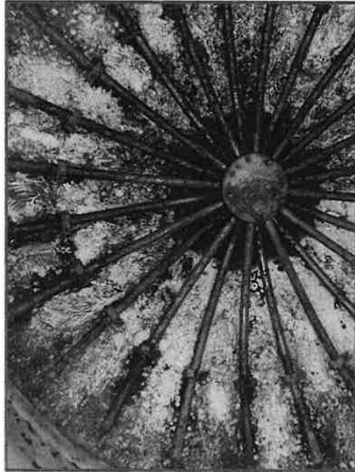
Figure 4: Close-up of stainless steel underdrain laterals and supports.
