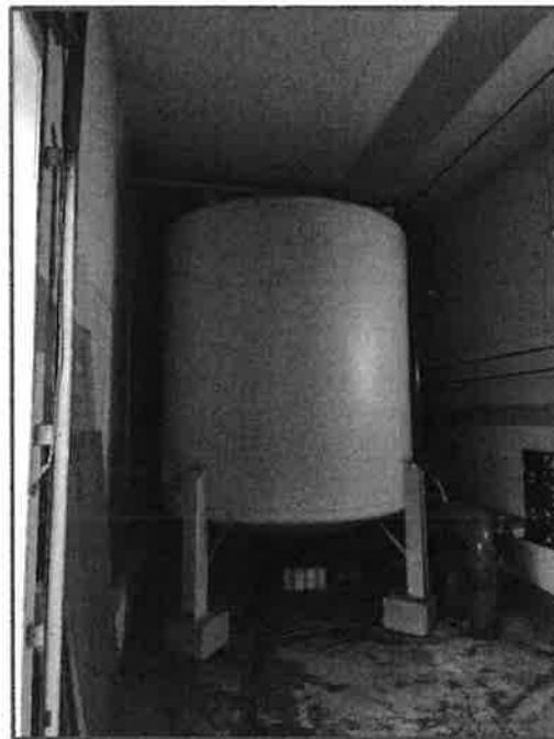
Figure 1: GAC Contactor #1, Units 2 and 3 are behind the unit shown.
