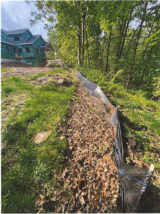
Figure 1: Eastern section of silt fence needs to be re-staked.
