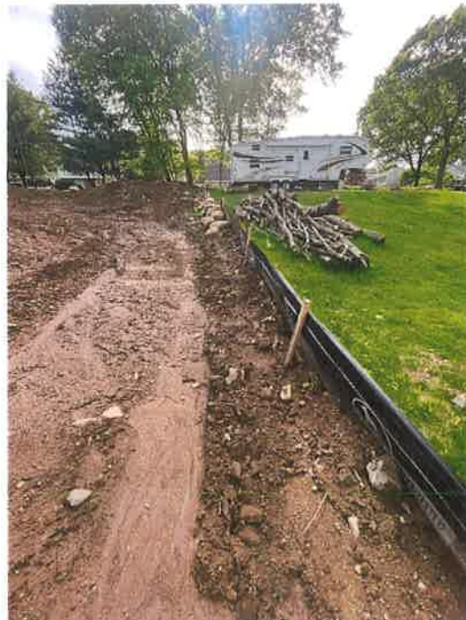
Figure 6: Northern section of fence collapsed.
