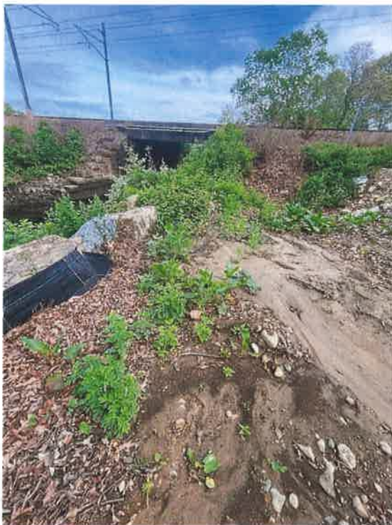
Figure 1: Silt runoff visible at southeast corner of the property.
