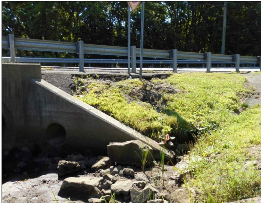
Photo No. 8 – Erosion at Southwest Embankment
