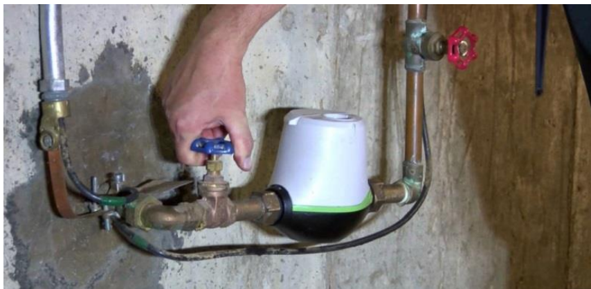
Figure 1 Newly installed iPERL meter
