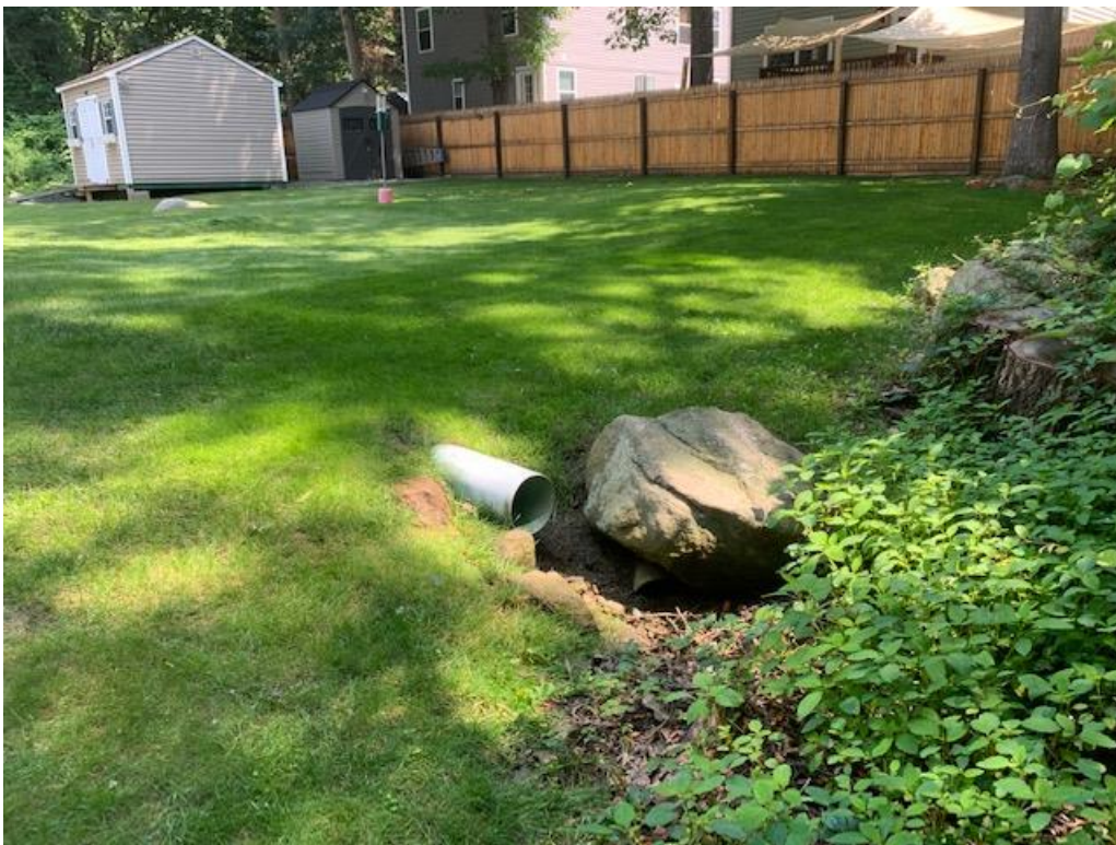
Photo 2: 8" Drainpipe that discharges to wetlands from neighboring property to the north.
